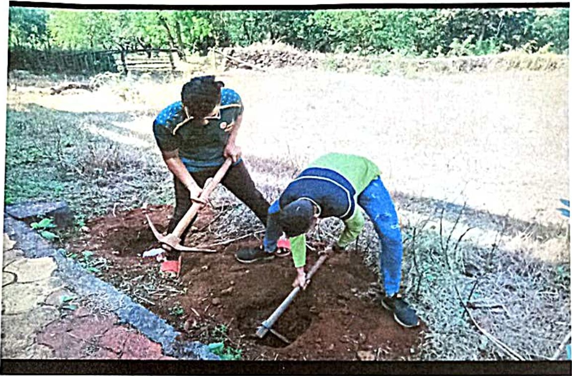
Waste dumping small puddles for wet and dry waste
